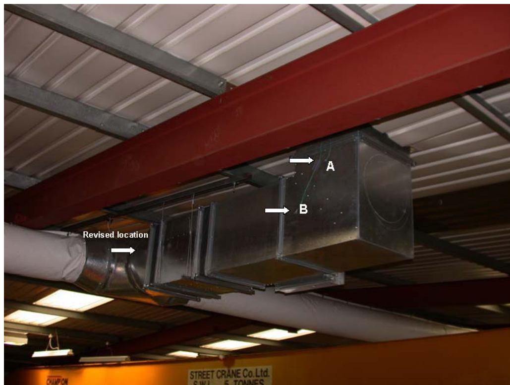
Figure 5 Location of thermocouples in duct within building
