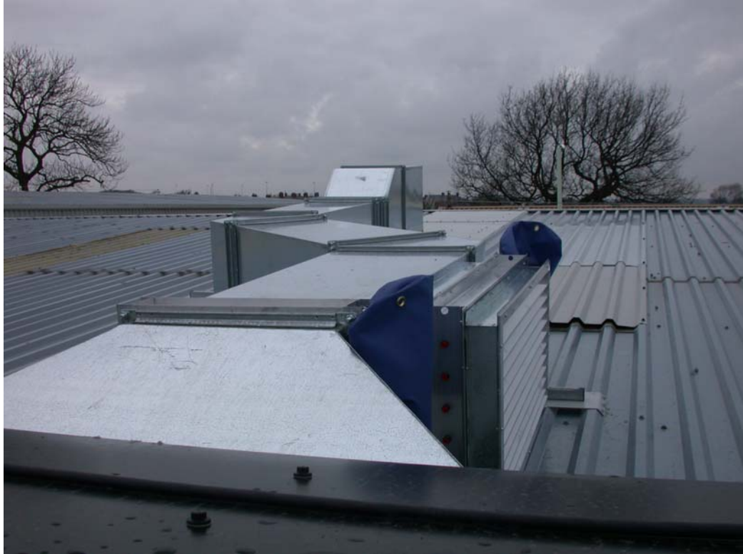
Figure 4 Duct from SolarWall™ to roof penetration
