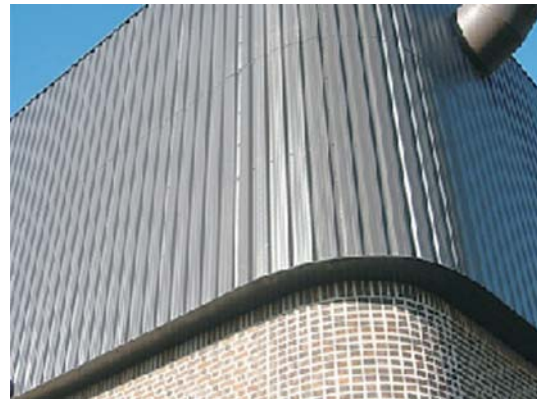
Figure 2: A completed SolarWall™
