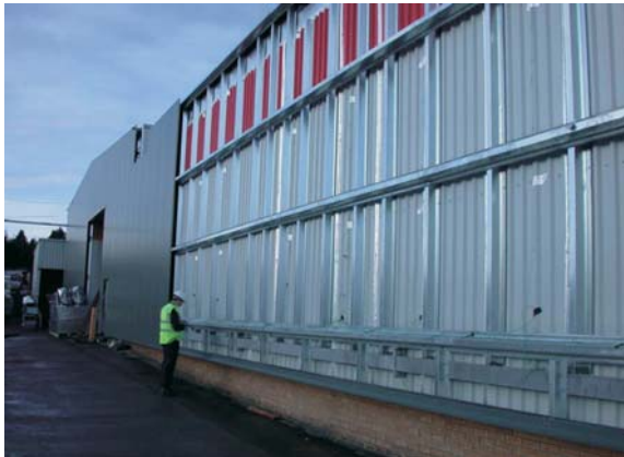
Figure 3: SolarWall™ showing thermocouples before placement of sheeting
