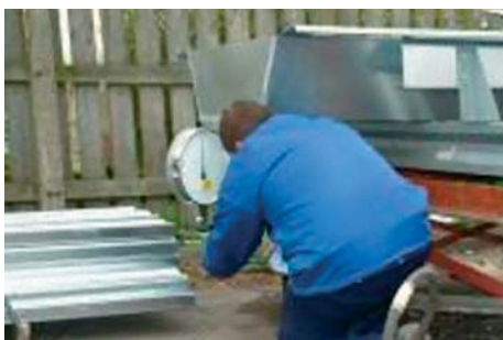
Test gauge connected to test piece outlet
