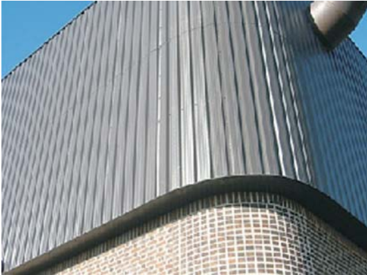
Figure 2: A completed SolarWall™
