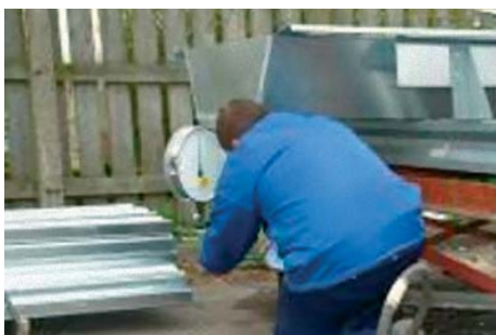
Test gauge connected to test piece outlet
