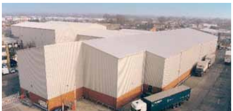
Figure 16. Refurbished building after pre-finished steel roof over cladding and the inclusion of improved insulation
