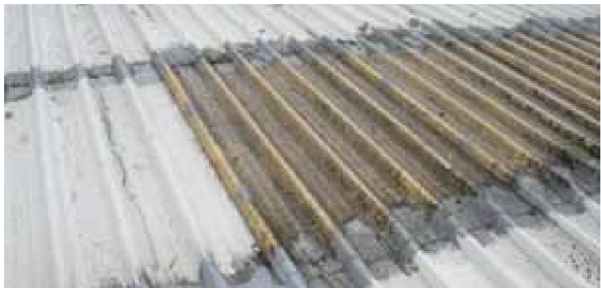
Figure 17. Before refurbishment showing failed roof cladding
